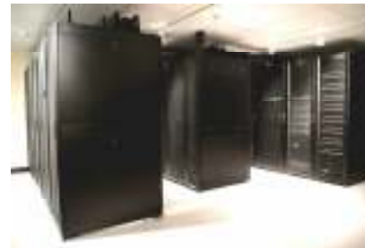
CIS X-Helion Data Center
